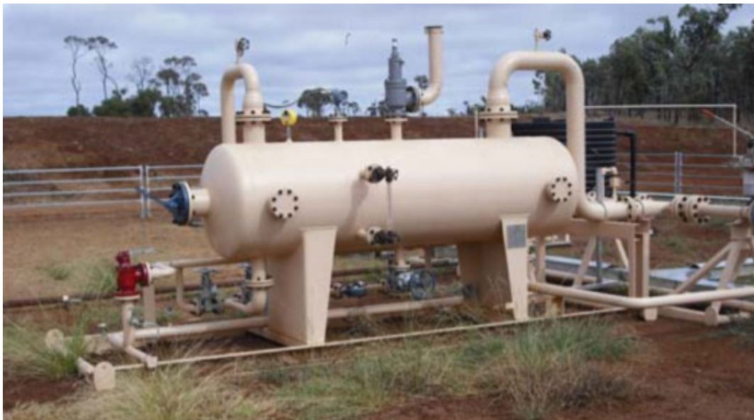
Figure 1 – Example Gas / Water Separation Equipment
