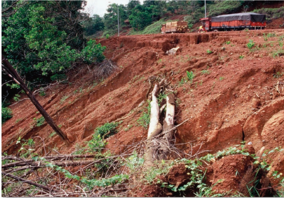
Figure C.7.12 Severe erosion of embankment material
