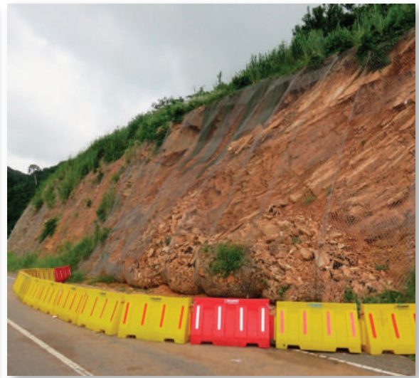
Figure C.7.2 Rock slide debris into road reserve due to sliding along adverse joints
