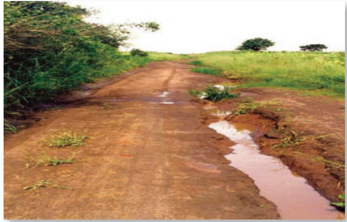
Figure C.4.16 Poor drainage in flat terrain
