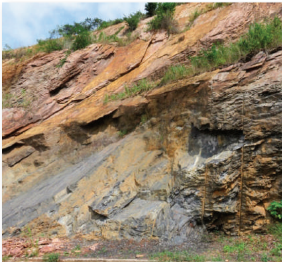
Figure C.7.1 Adverse jointing in rock slope prone to sliding along smooth joint surfaces
