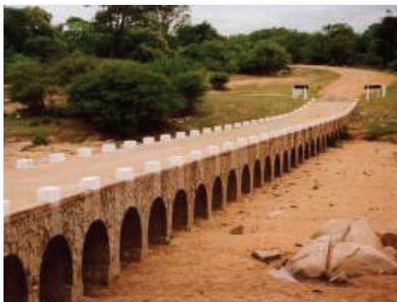
Figure C.4.13 Large vented causeway
