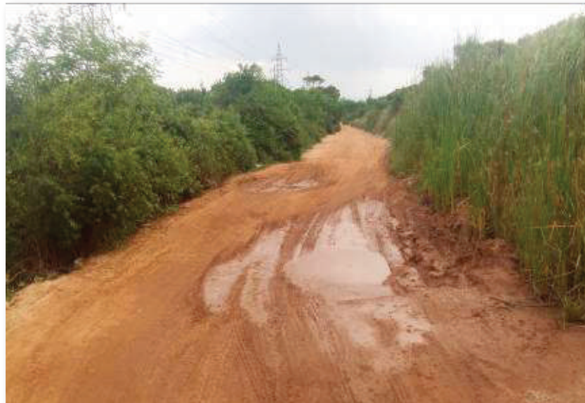
Figure C.8.2 Stagnant water due to poor camber
