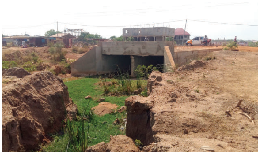
Figure C.6.7 Erosion of channel at downstream of culvert
