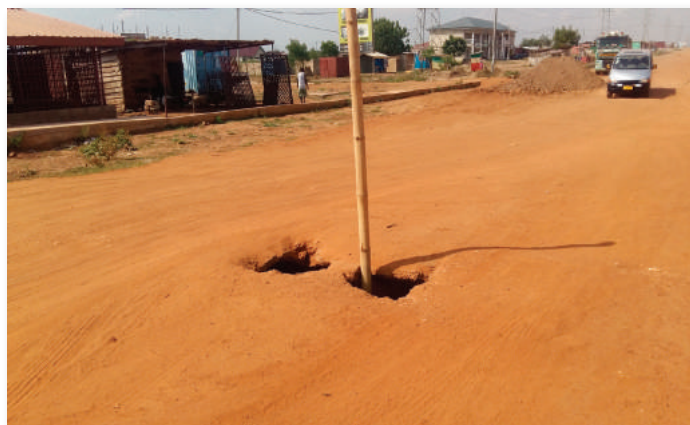
Figure C.4.8 Damage to a pipe culvert due to inadequate cover
