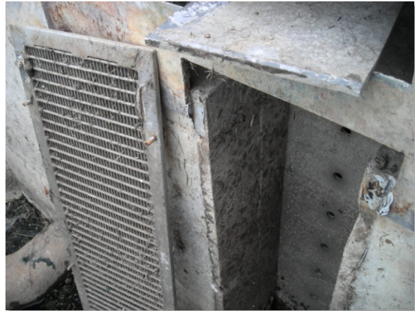
Photograph OS-2. This trash rack could not be properly attached due to its inadequate flange width.
