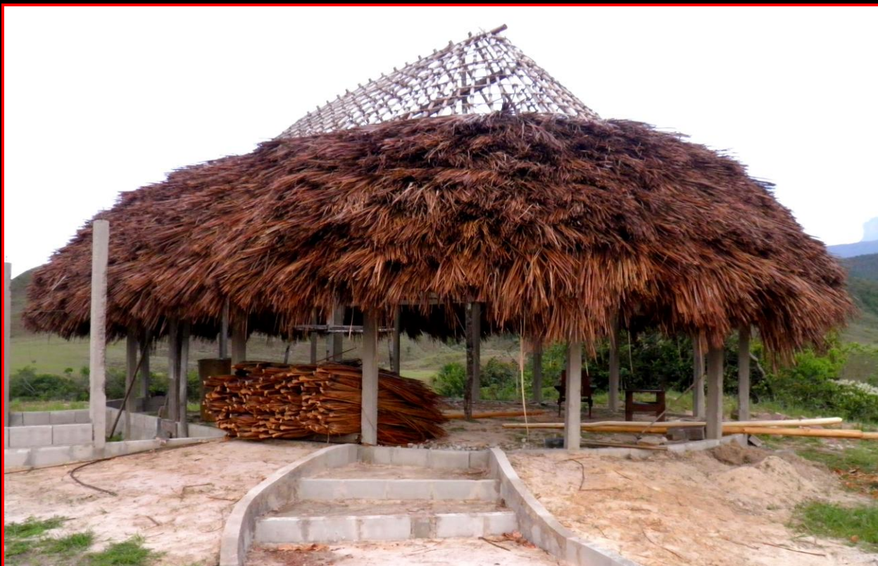
Kavac assembly hall under construction. Quality palm frond roof construction is good for about twenty years. Photo: Marianela Camacho, 30 June 2012
