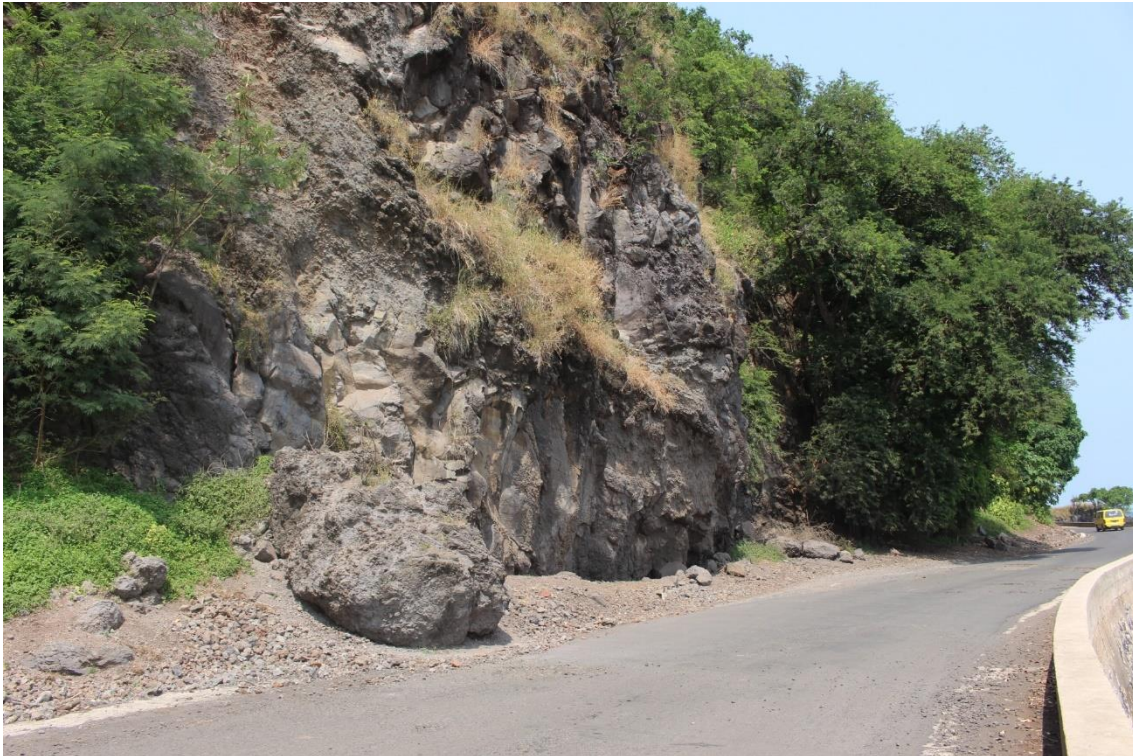
Figure 4-11: A dangerous slope (combination of causes)
