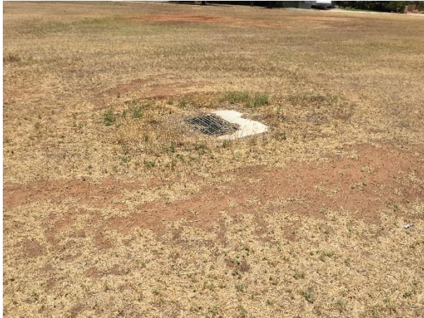
PLATE 7 – Stormwater infiltration area (grate with retention depression).
