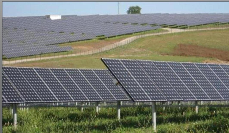
Figure 3: A PV solar panel array similar to that proposed for the project
