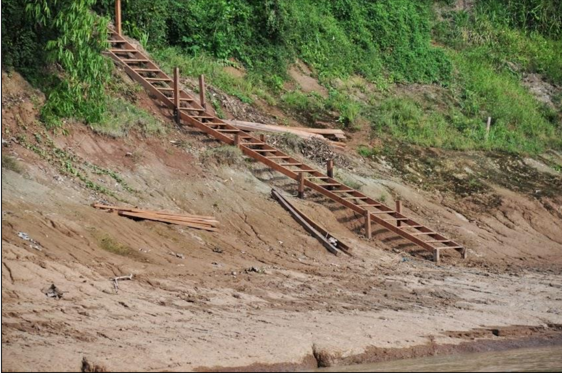
Stairs Built at Purus Project for Mr. Benedito (Photo Credit: Brian McFarland)
