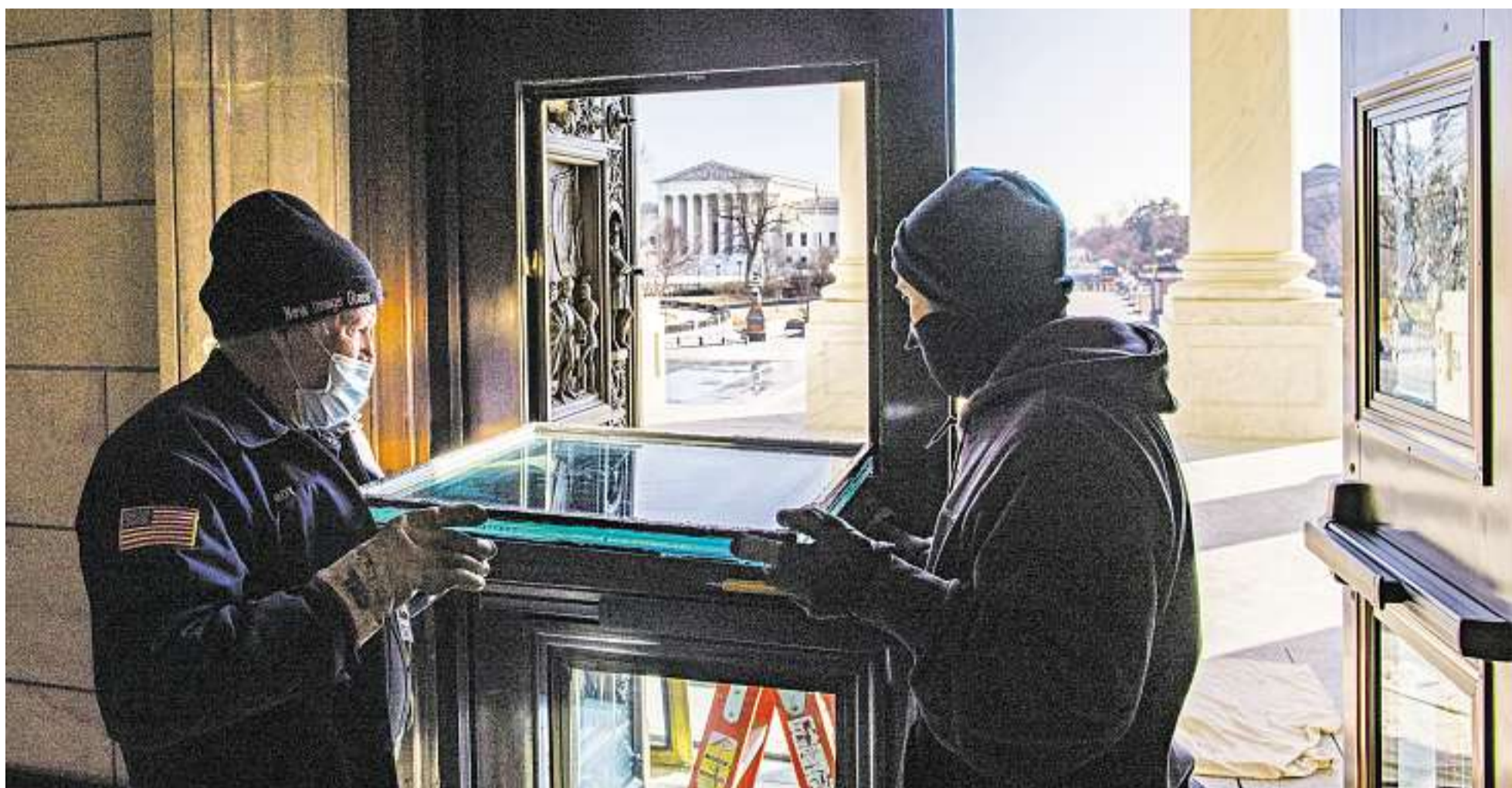
Workers on Monday repair glass on the East Front rotunda doors that was damaged during the deadly Jan. 6 assault at the U.S. Capitol.
