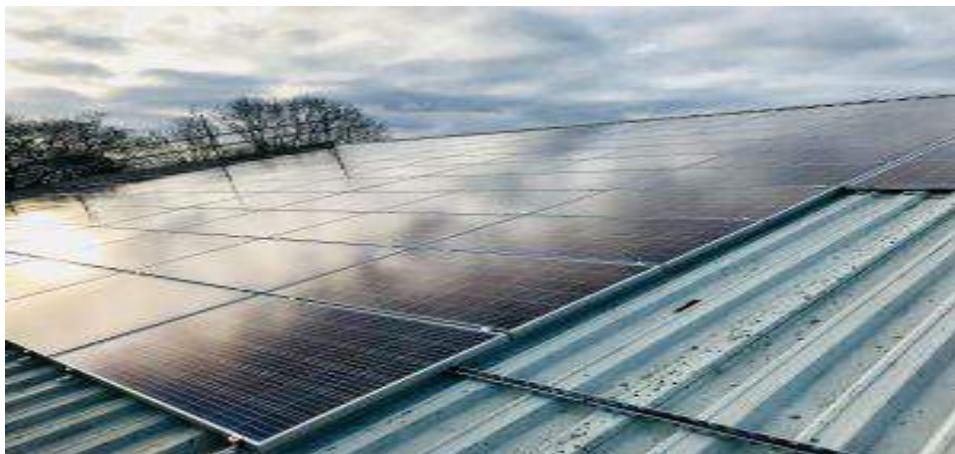
Solar panels on Woodford Park Leisure Centre
