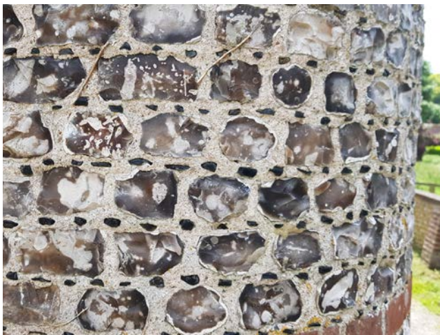
Galletting, where small pieces of stone, tile or brick are pushed into the wet lime mortar
