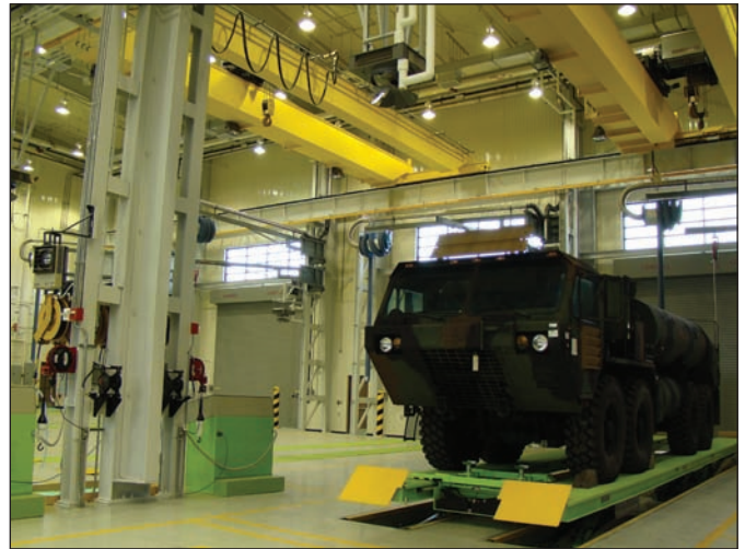
The picture shows the inside the newly built Pfc. Melvin L. Brown Maintenance Facility on Camp Carroll. The facility features 16 maintenance bays of each can fit two medium trucks or up to four Humvees. (Photo by Kim Chong–yun)
