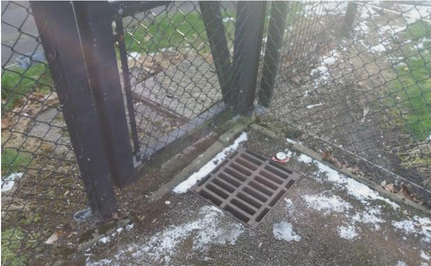
Fig 3: Tennis courts drainage outlet grate
