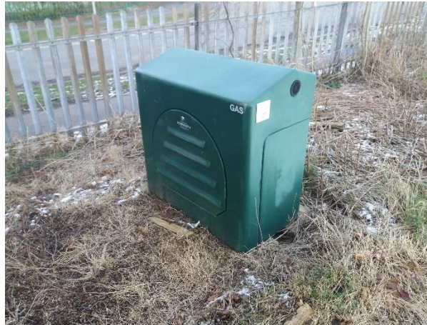
Figure 2: Gas infrastructure within the site boundaries needs identifying prior to improvement works commencing.
