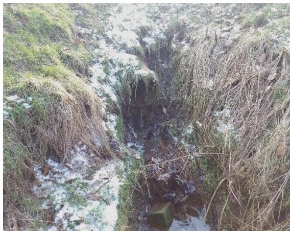
Figure 4: Culvert pipe at the sites Northern end discharging from an unknown origin towards the brook.
