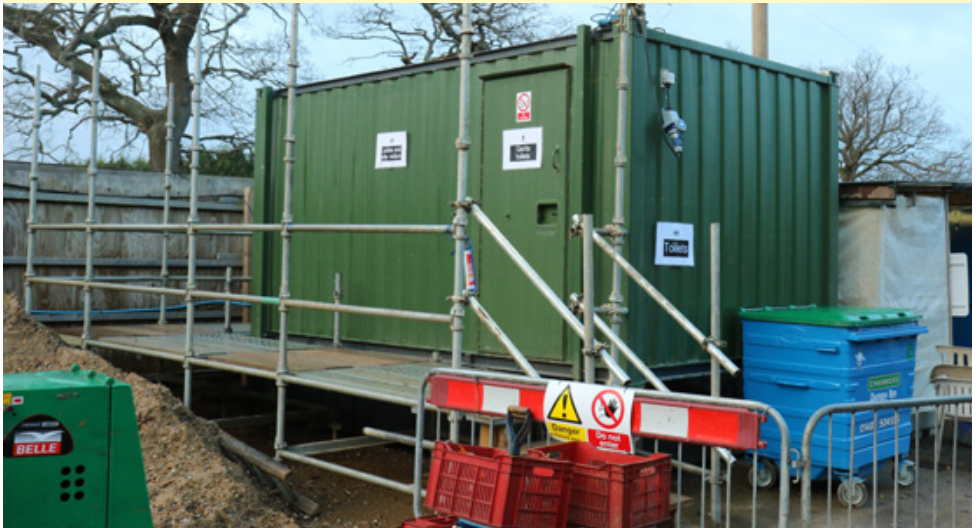
Below: Not the most glamorous item on the Trust's equipment register, but a useful investment – a second-hand 'sanitary facility' now installed in the work compound at Compasses and scheduled to move to other sites in the future.
