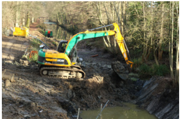
Destined for the Burnsife - Andy Evans and the digger remove more of the dam from the north side of Compasses Bridge.
