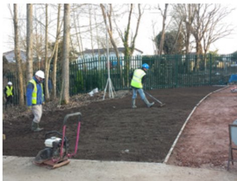
21st January 2017: Landscaping work in progress - Compasses Bridge is in the right-hand background.
