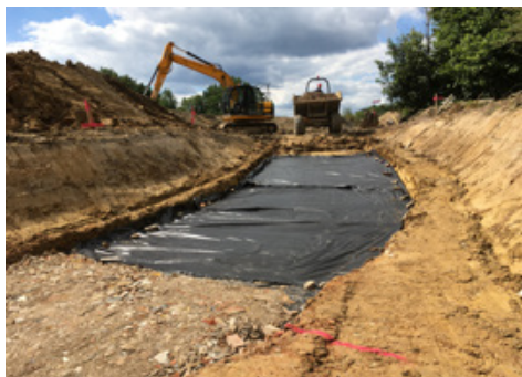
Construction work is in progress on the slipway during the WACT Summer Camp in July 2016. (Adam Morris)
