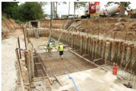
August 2015: Contractors are pouring concrete to form the base of the new Gennets Bridge Lock.
