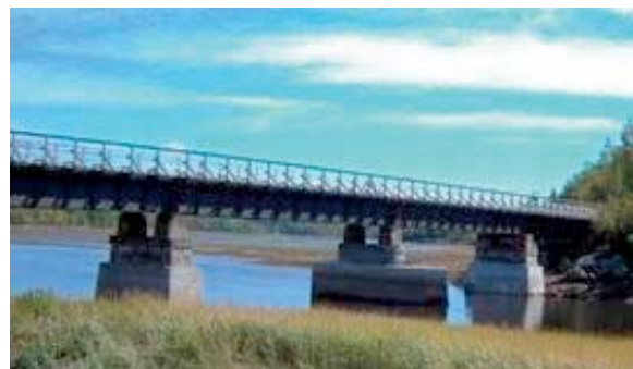
French River Bridge in 2010 showing completed repairs to concrete support piers. Funding was provided by NTC / Government of Canada, Government of Nova Scotia and the Municipality of the County of Colchester.
