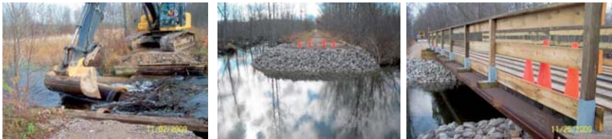
Removal of a condemned bridge and construction of a new 50 foot long Black Creek Bridge on the North Simcoe Rail Trail near Wasaga Beach in November 2009.
