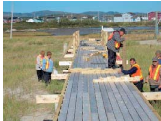
Construction of a boardwalk in 2009 on the Grand Bay West Trailway in Port-aux-Basques.
