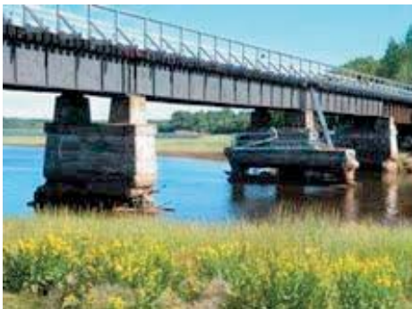
French River Bridge near Tatamagouche in 2009 as repair work was commencing on the eroded centre support pier. Photos courtesy of Bob Gould, Tatamagouche Area Trails Association.
