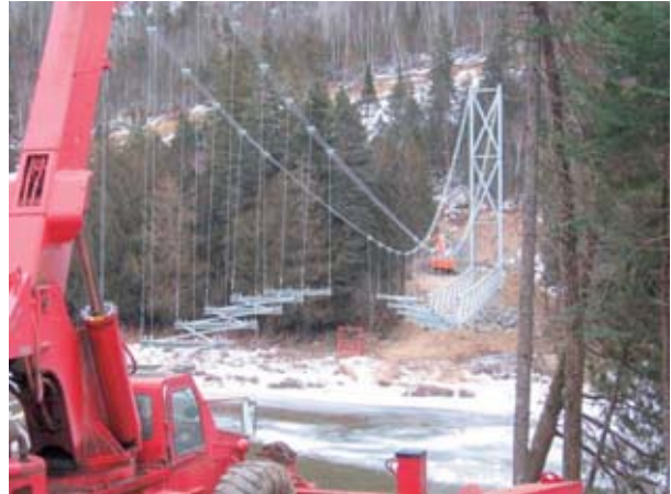
Construction of the Grande-Rivière Suspension Bridge in the Gaspé Region of Quebec in 2009.
