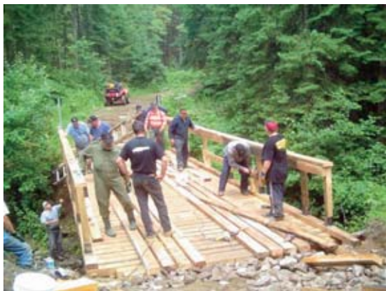
Rehabilitation of the Salarno Creek Bridge near Lakefield. This was a joint project of two local off-road motorcycle and snowmobile clubs.
