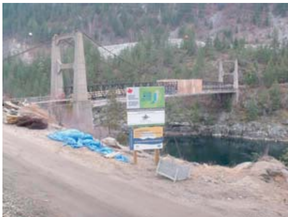
Restoration of the Brilliant Suspension Bridge over the Kootenay River near Castlegar.
