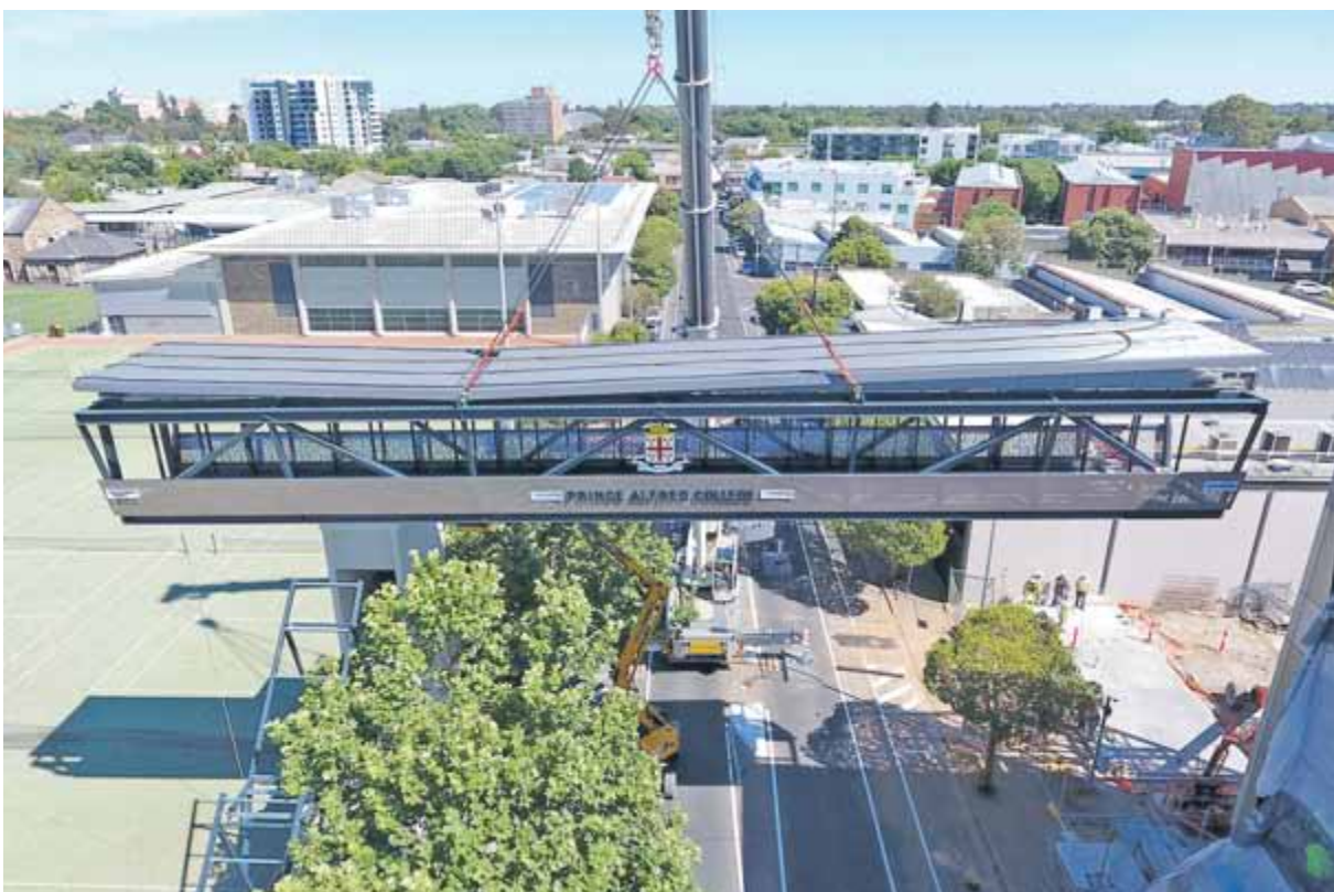
THE BRIDGE... Putting the new bridge in place was a delicate operation.
