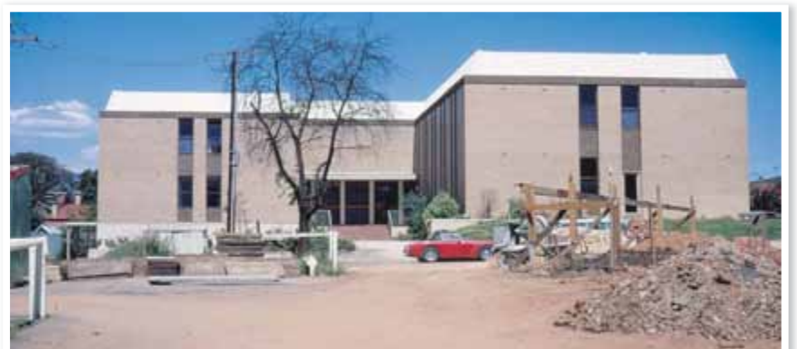
FIDDIAN WING... Known then as Pirie, with construction of The Chapel commencing in the foreground.
