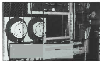
The Gas Station's state-of-the-art blending panel can supply; enriched air nitrox, heliox, trimix, oxygen and argon to your specifications.
