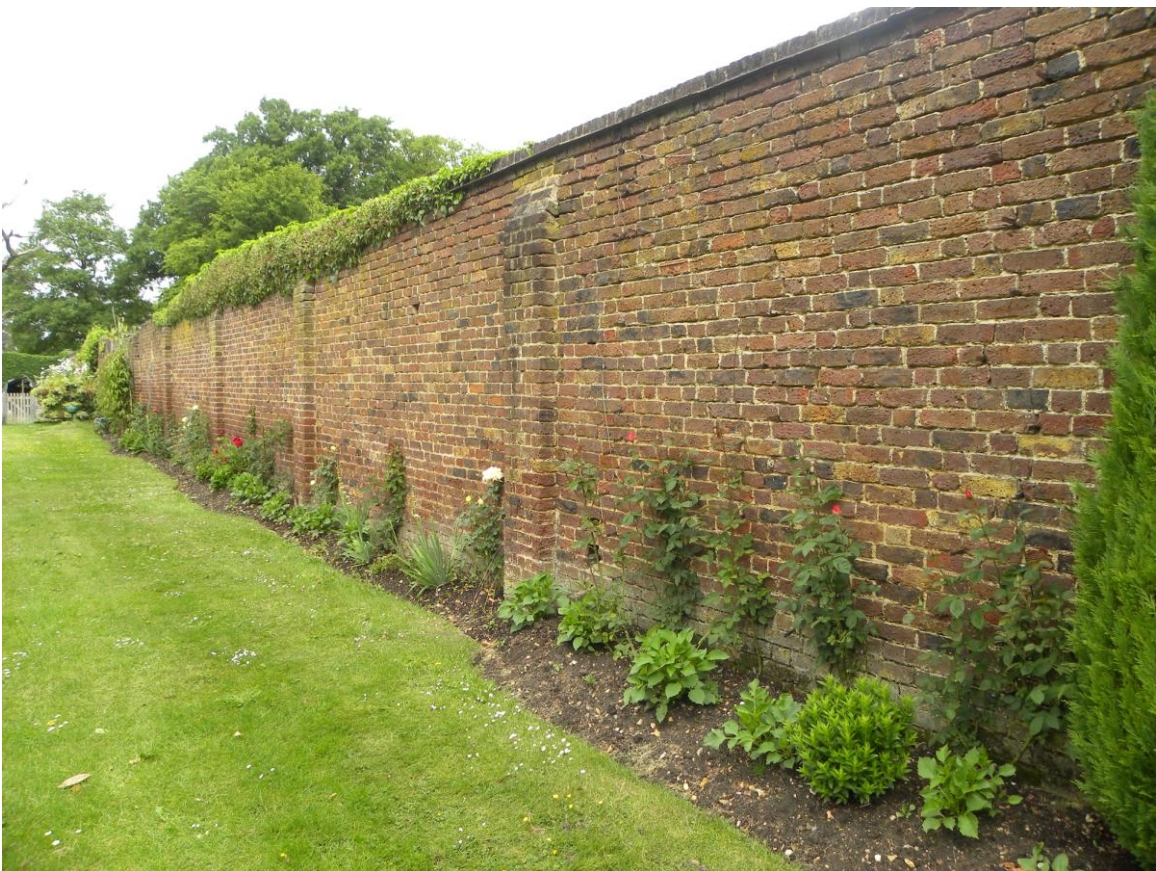
Looking west along the wall which would have formed the back of the long glasshouse, and facing south to take advantage of the sun.
