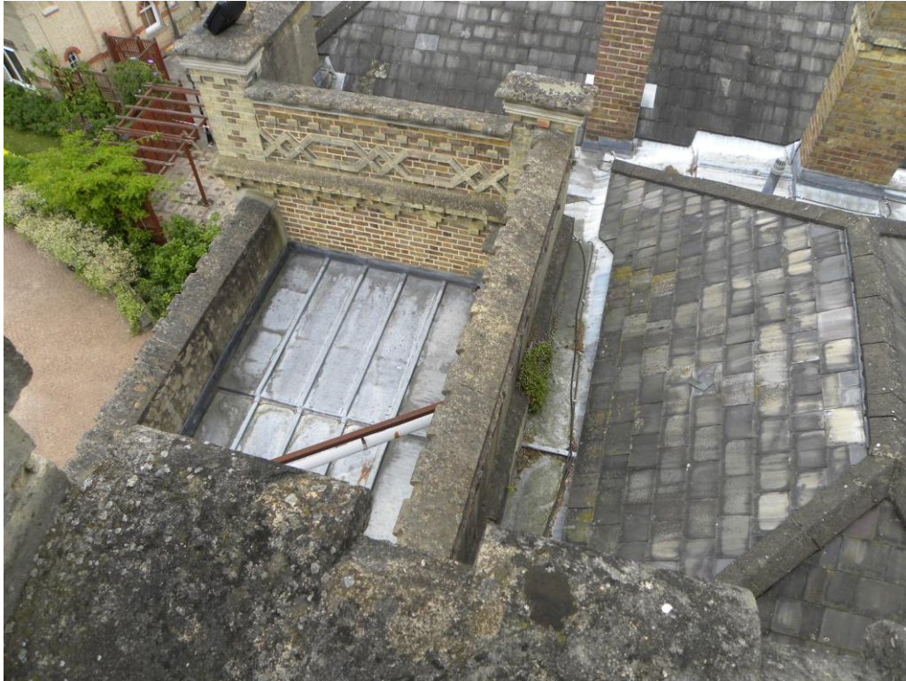
Looking from the roof of the tower in a westerly direction. The flat, leaded roof of the extension to the south front can be seen on the left and contrasts with the hipped, slate roofs of the original building.
