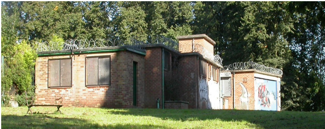
The pavilion building has suffered from sustained vandalism
