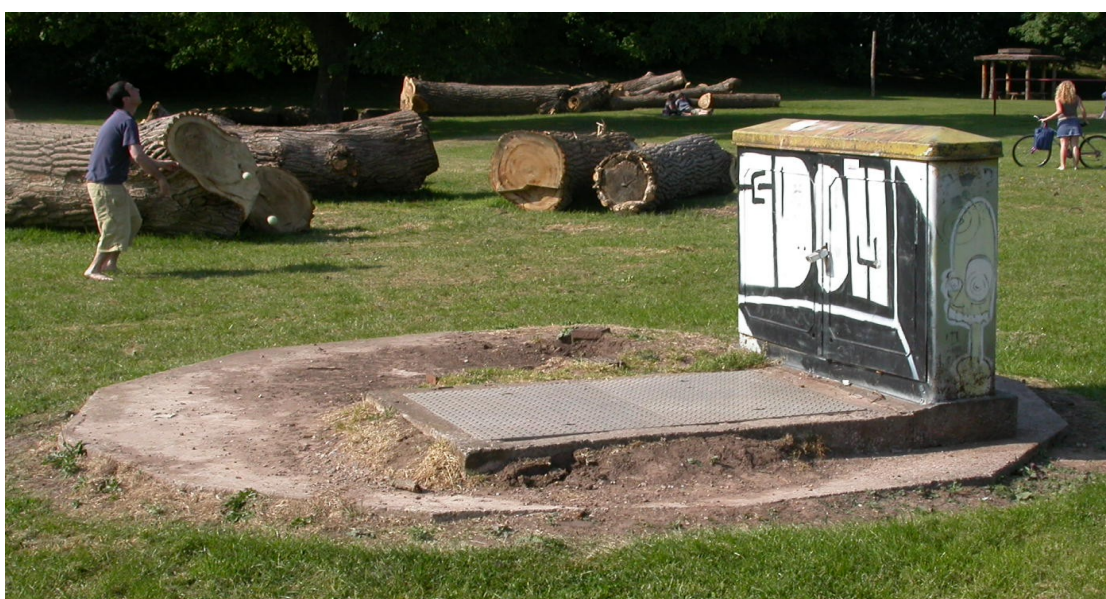
Part of the underground pumping system located within the park
