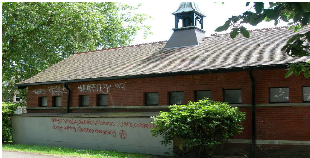
Other buildings in the park have suffered from graffiti damage
