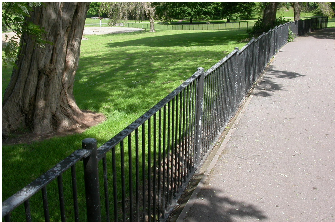
The condition of internal boundaries needs some improvement
