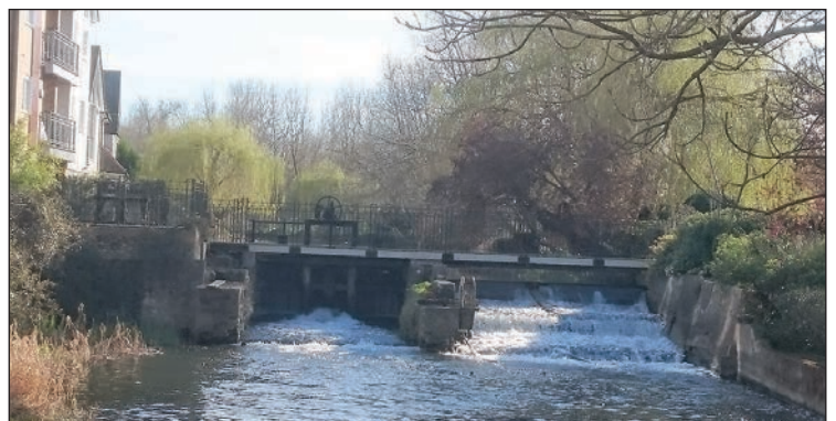
Weirpools can also be oxygen depleted
