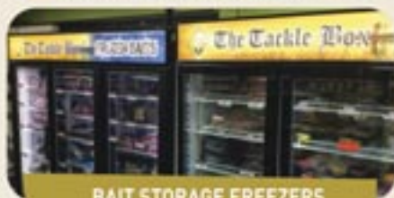
BAIT STORAGE FREEZERS
