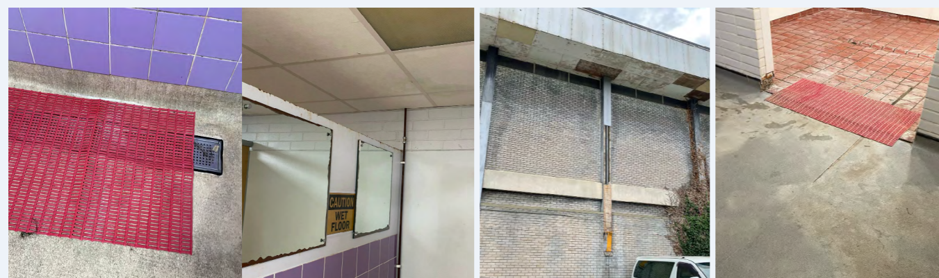
WET CHANGING ROOM FLOOR CONDITION | LIGHTS OUT | MIRROR DAMAGE | EXTERNAL CONDITION WATER DAMAGE | DAMAGE | DRY CHANGE TILE & FLOOR DAMAGE
