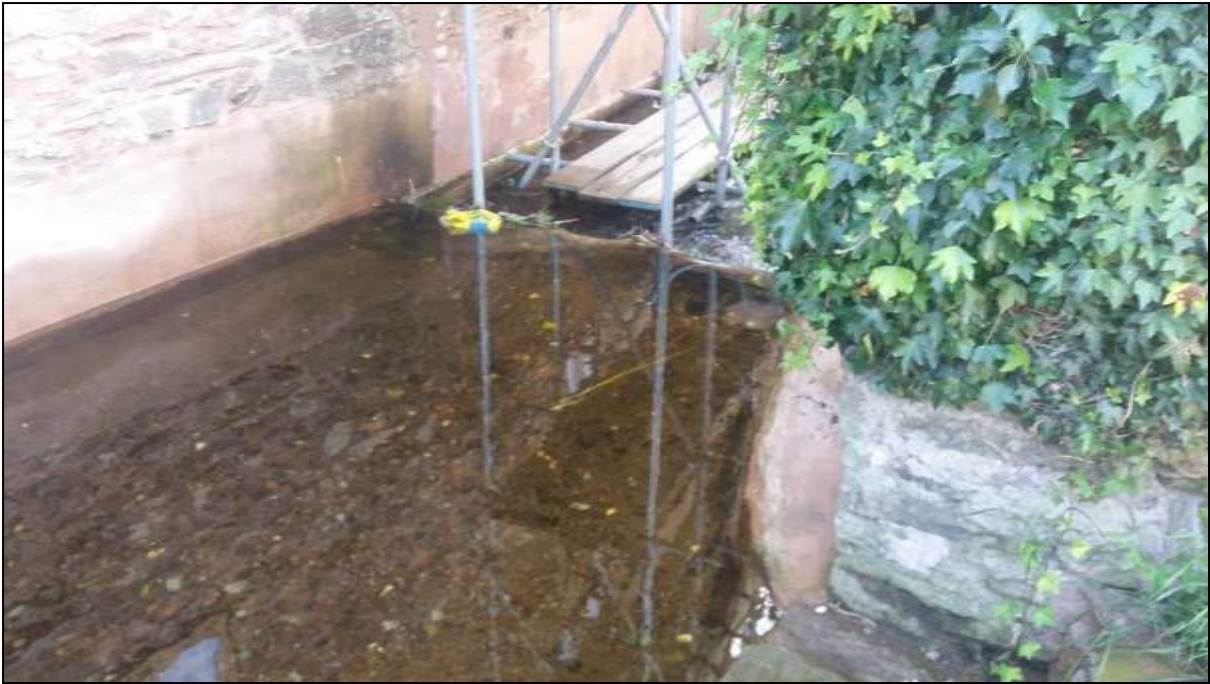
Figure 9: A small stoplog in the river should be removed
