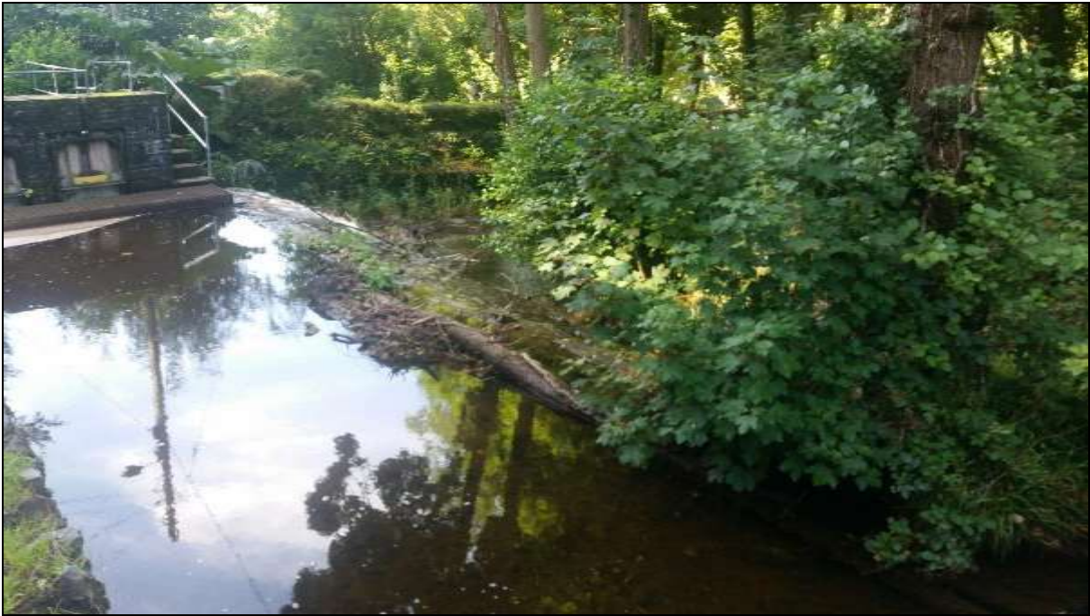
Figure 21: The 7m section of weir next to the sluice diverts excess flow around the island
