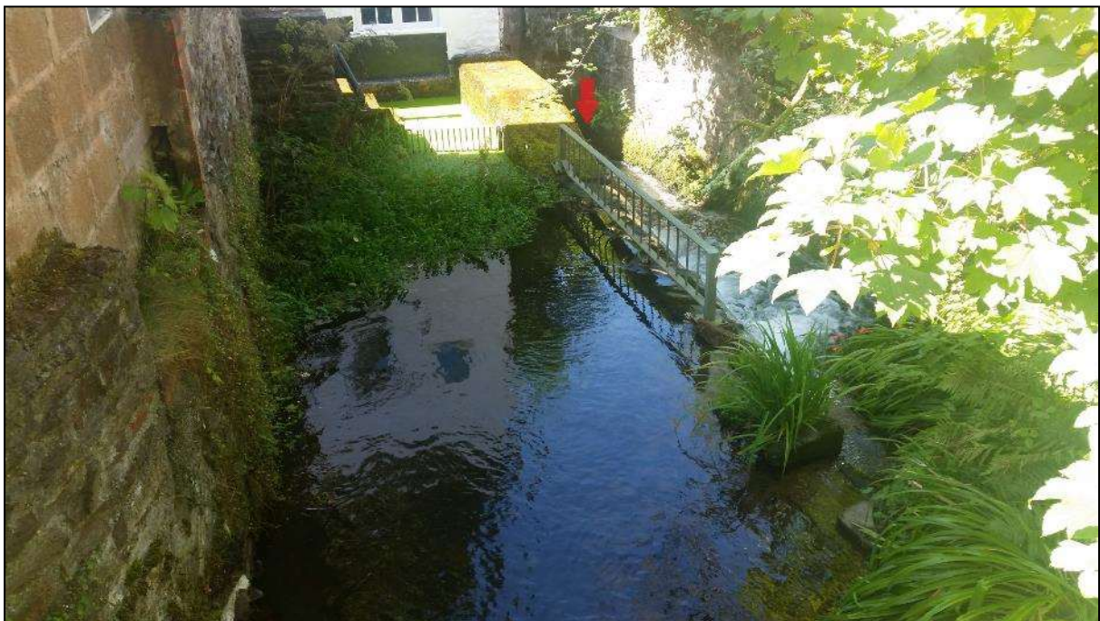
Figure 4: The entrance to the culvert (red arrow) is below an old mill weir
