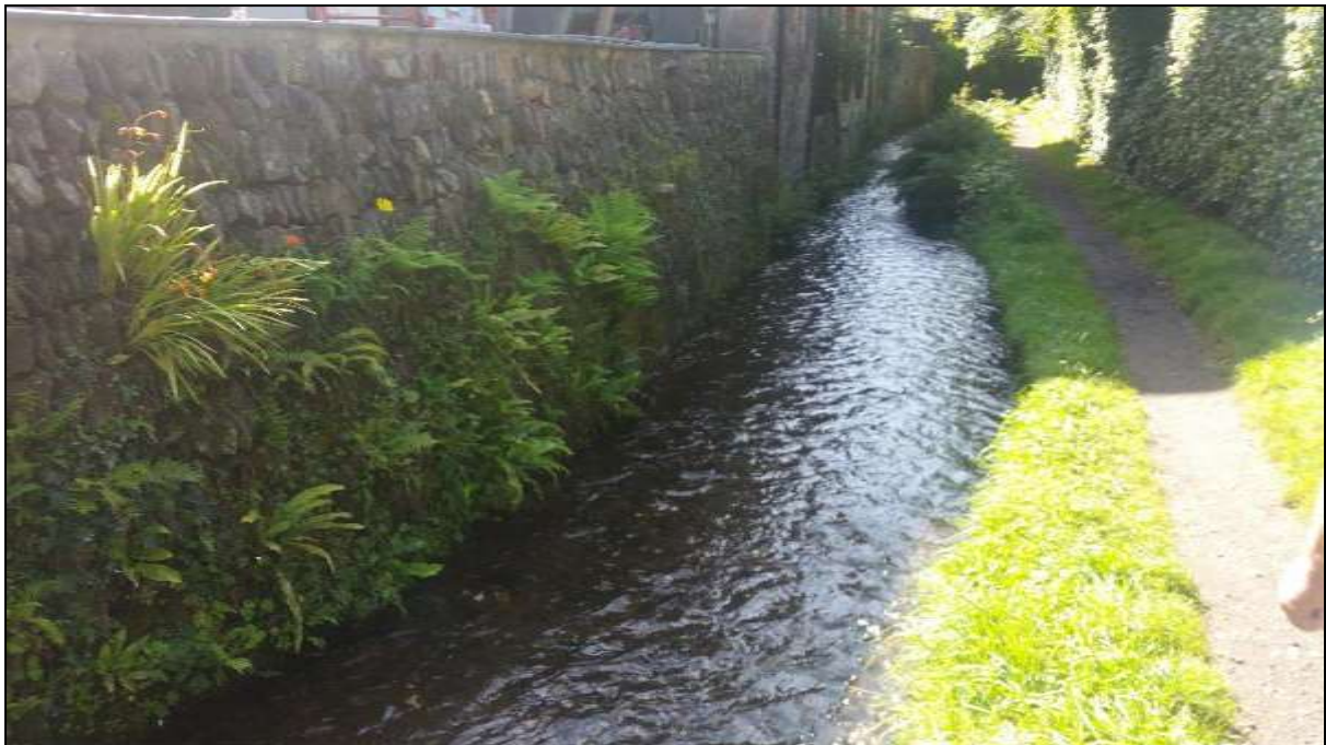
Figure 12: The tall wall on the LB colonised by a few ferns but otherwise providing very little habitat
