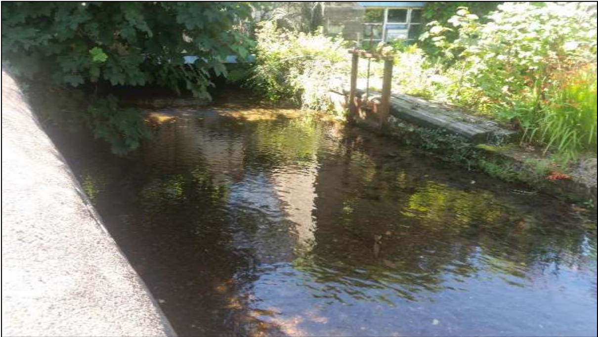
Figure 5: The riverbed above the weir has risen as sediment has accumulated. When the mill was in operation the sluice pictured would have regularly diverted flow through a secondary culvert and flushed the channel
