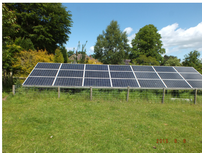
Solar Panel Array - Sandiway Photo Courtesy of Stuart Middleton
