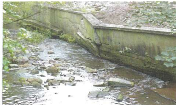
Collapsing retaining wall adjacent to Shelf Brook 29 June 2000
