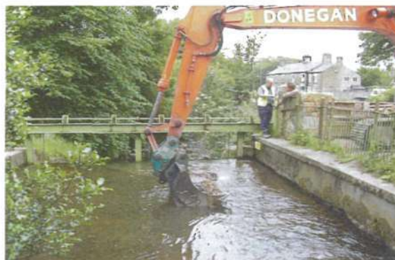
Excavation to the culvert on Shelf Brook 29 th June to create bypass channel.
