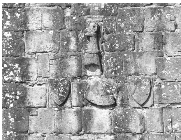
Fig.12.10: Heraldry above the south gate, Bodiam Castle. Dallingridge's helm above; below, two shields now blank, and between them the arms of Sir Robert Knollys Dallingridge's war captain in France and owner of Derval. Knollys' arms are couché or tilted (i.e. as carried by a mounted knight).
