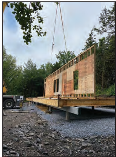
A CRANE LOWERS part of the frame of a new Habitat for Humanity home in Vergennes during a recent work day on the Booth Woods site. The volunteer-built home should be ready for occupancy by the Muir family of four early next year.
