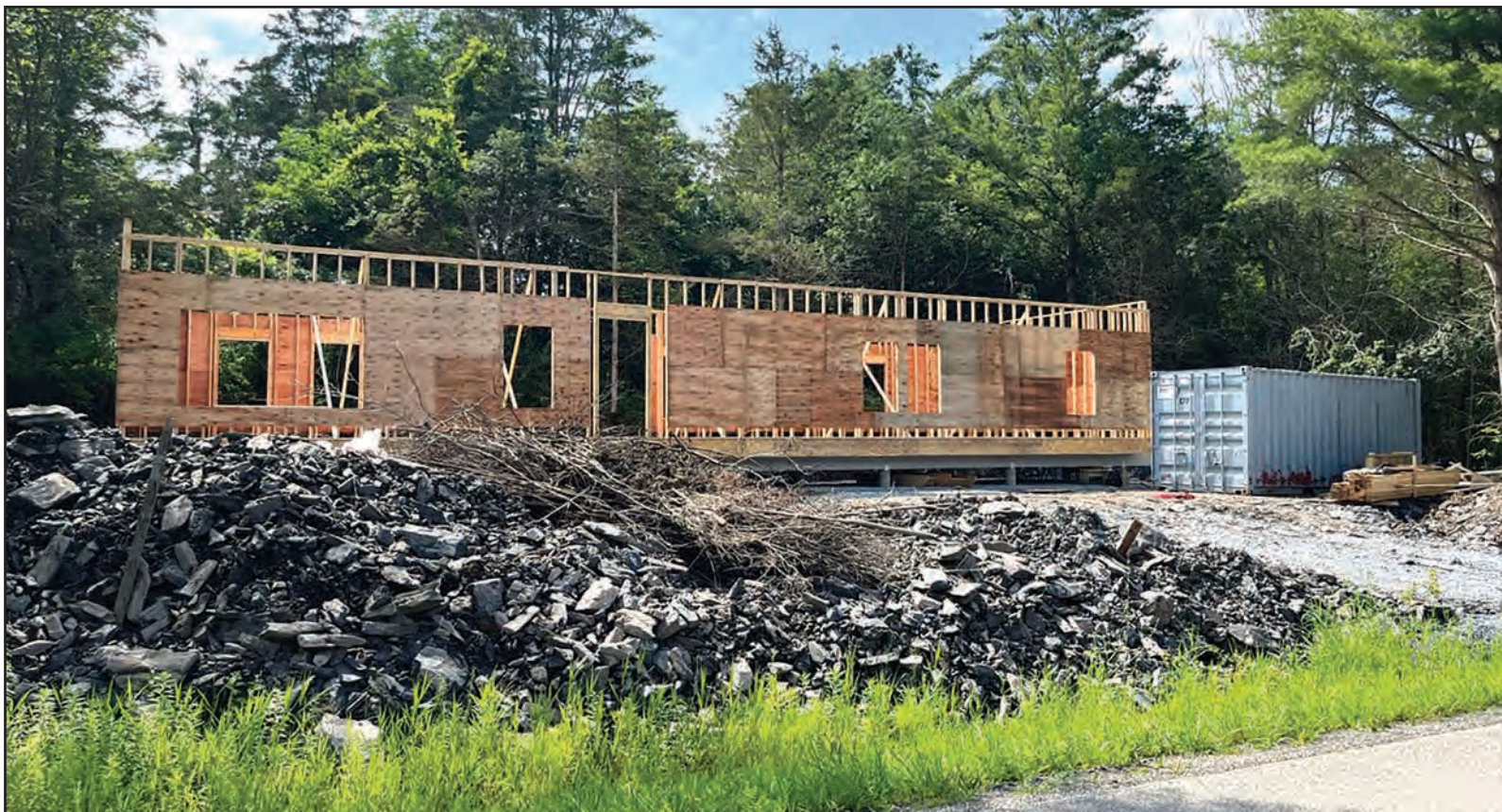
MUCH OF THE framing is in place for the Habitat for Humanity home in the Booth Woods neighborhood in Vergennes, which is projected to be ready for a family of four in early 2024.
