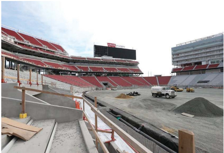
Construction work was completed in July and the stadium officially opened in August
