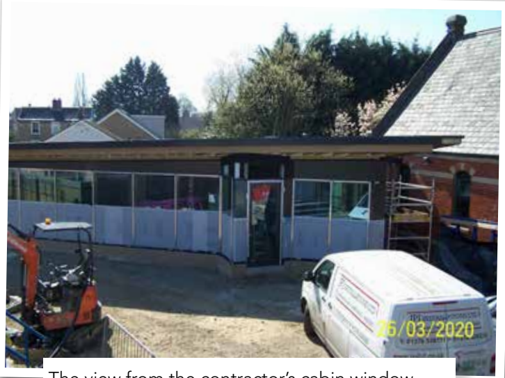
The view from the contractor's cabin window – glazing and main door in place under the roof which is now finished.
