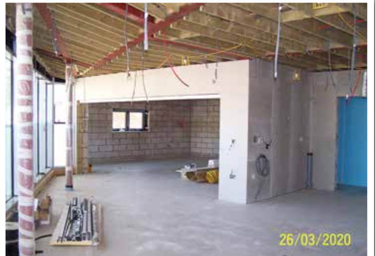
The new building as you walk through from the chapel; the meeting room is framed by the stud wall which will have a folding door. When not sectioned off for meetings, it can be incorporated into the café area, seen in the foreground. The kitchen & serve-over will be in the bottom right hand corner. Eventually.
