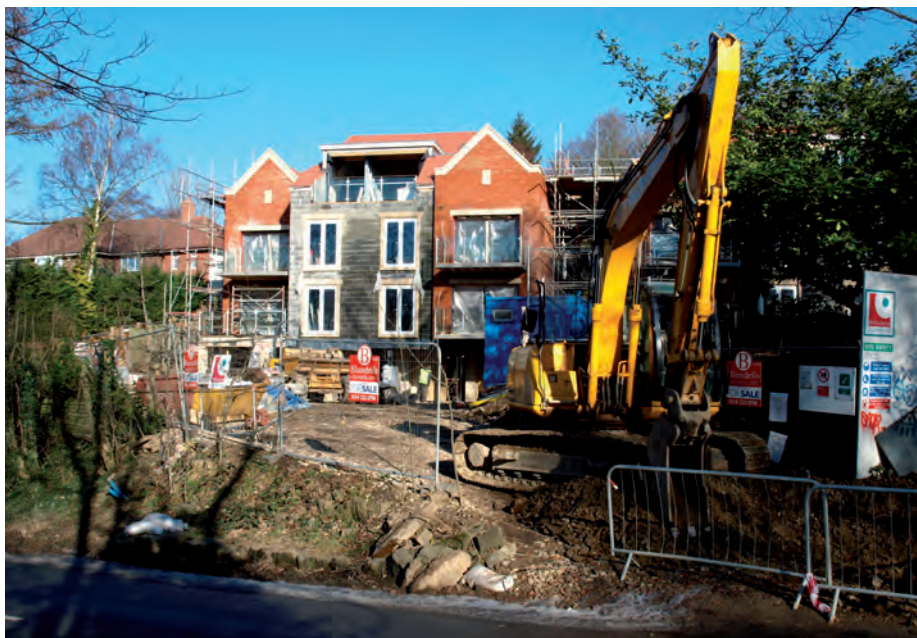
The new flats taking shape on Twentywell Lane. There are 10 units with lifts and secure parking and guide prices in the £250-350,000 range.
